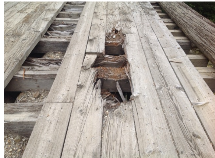
hole in deck
